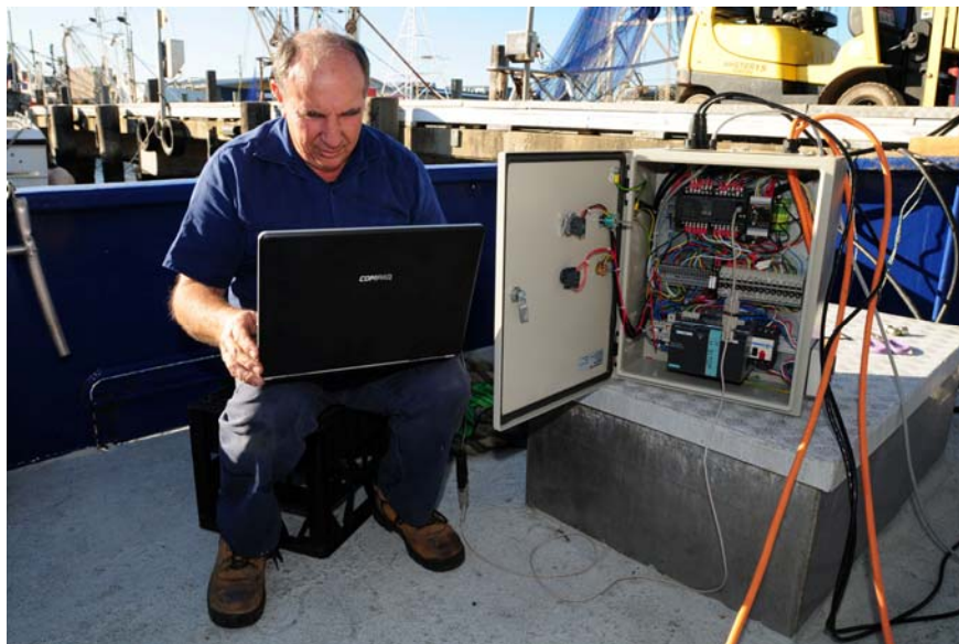
Engineer Peter Ashworth setting up the control box (right) by computer. The control box controls all the functions of the underwater setter, including speed and duration of cycling and transmission of functions to vessel VMS, which is an essential component of monitoring compliance.
